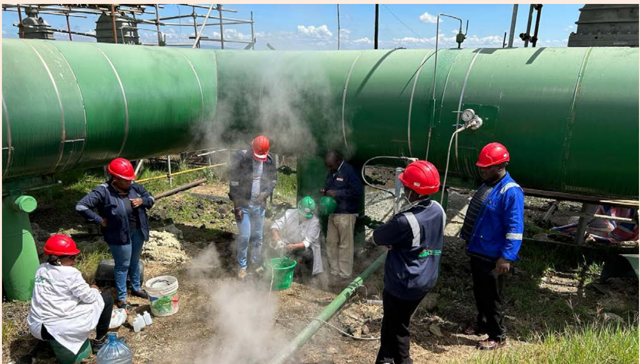
Collecting samples to assess steam purity. Menengai Commissioning Assistance project supporting GDC in Kenya. Credit: JRG Energy/Kevin Brown.
