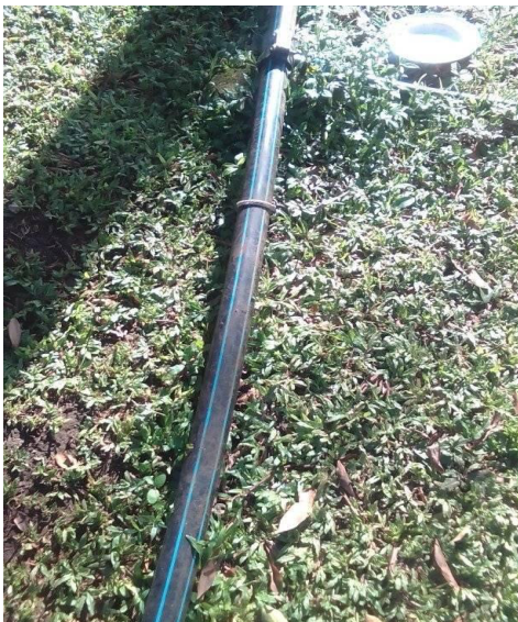
Figure 20: Example of exposed water pipe, photo taken in Sanma province
