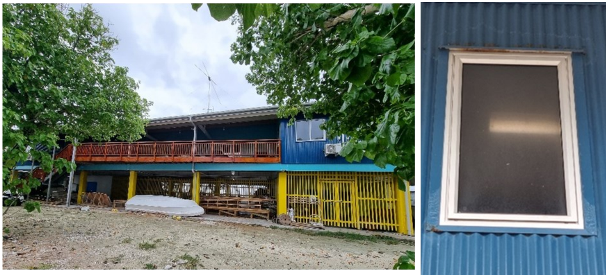
Figure 7: New Zealand-funded fisheries building opened in 2019, with example of rust degradation (right)
