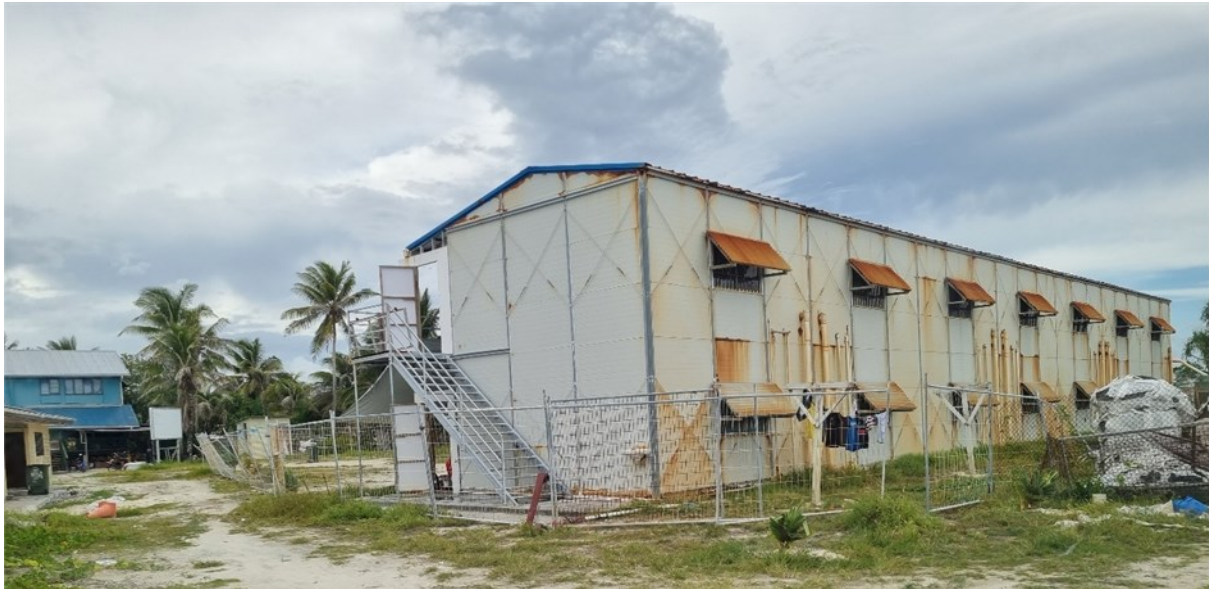
Figure 8: Other building completed in 2019 with evidence of early decay
