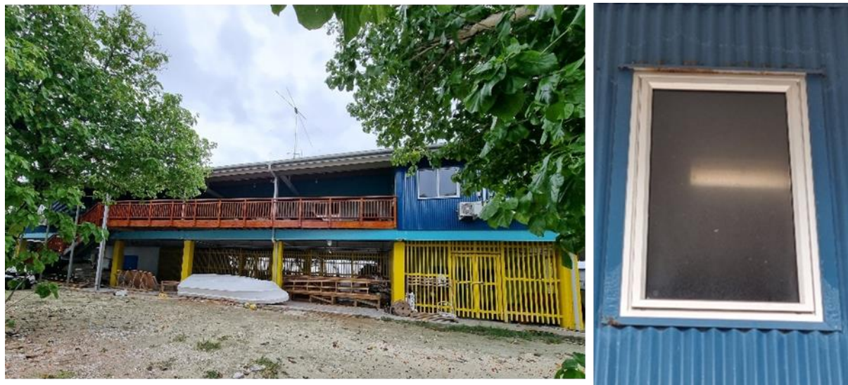
Figure 7: New Zealand-funded fisheries building opened in 2019, with example of rust degradation (right)
